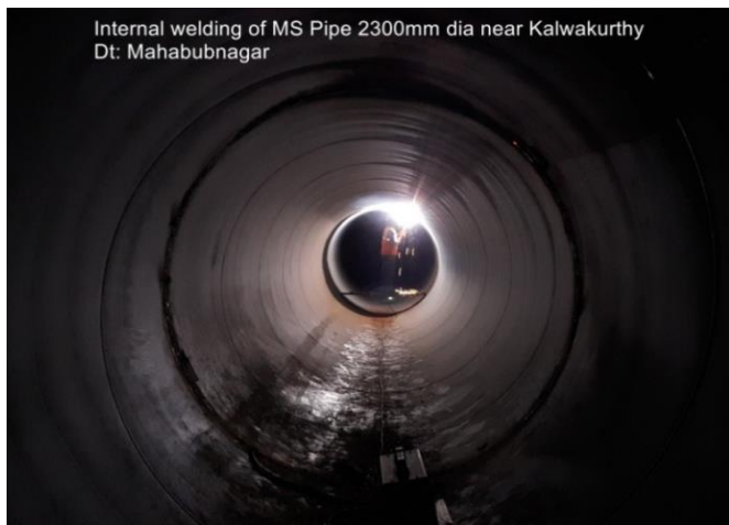
2.4 mtrs dia MS Pipe line
