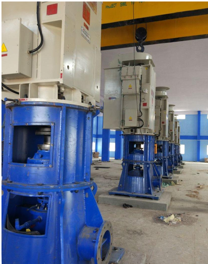
Pumpsets @ Mallannagutta WTP
